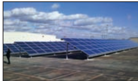
Ground mounted solar array at Kastle Technologies.
