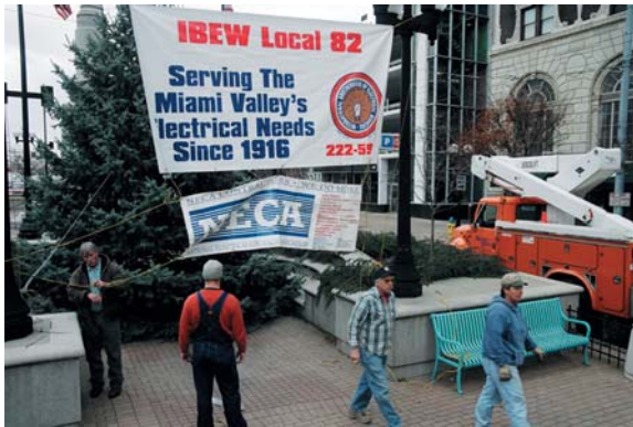
Thanks to NECA contractors Chaple Electric, Newco, Wagner Smith and Studebaker Electric for volunteering their time and equipment to light up the city.
