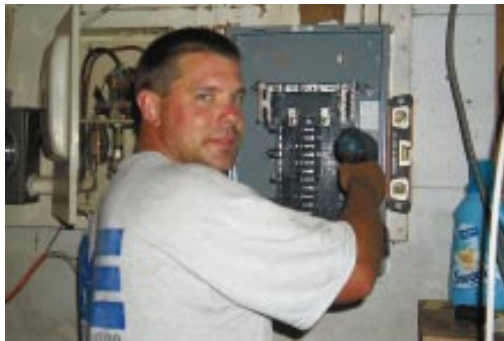
IBEW Local 82 Journeyman Scott Daniels, with Mutual Electric, installs a new breaker panel.
