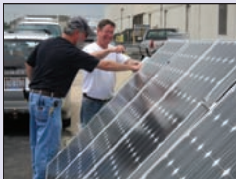
Journemen Kenny Westendorf (left) and John Rienert learn to install solar panels.
