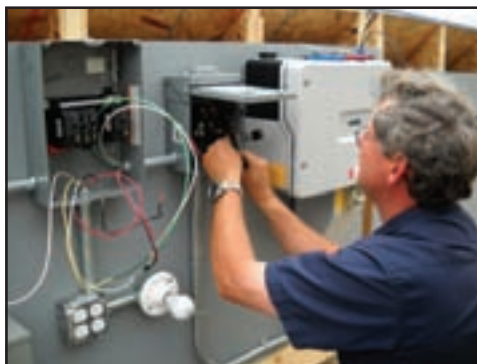
Bright Street Superintendent Jim Blair connects the solar array to the grid.
