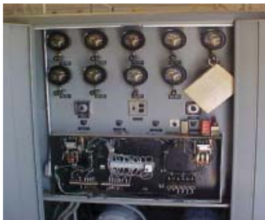
Oil pressure system, Area B, WPAFB. Rebuild by ESI.
