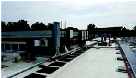
Inverters at KMS.
