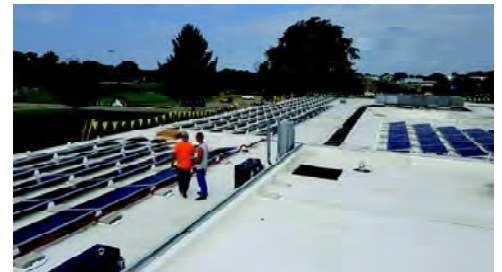
Solar installation in the South Unit.
